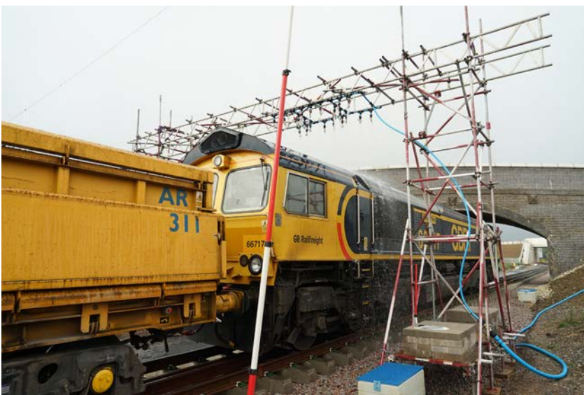
Dust suppression system at Charbridge Lane
